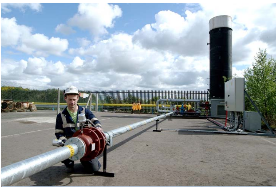
Riccall Mine, enclosed stack flare and flame arrestor
