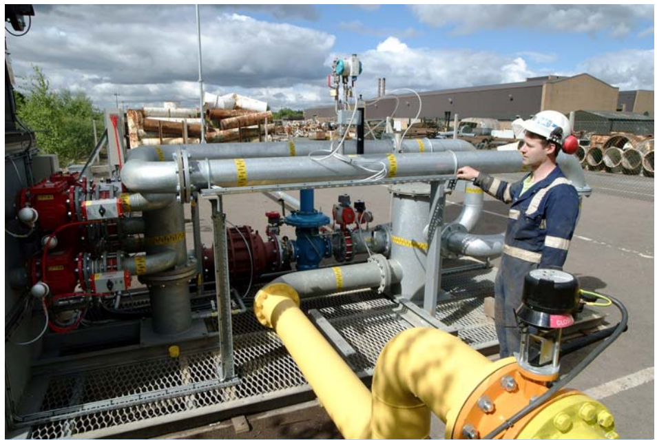
Riccall Mine, flare safety and monitoring equipment mounting in pipeline
